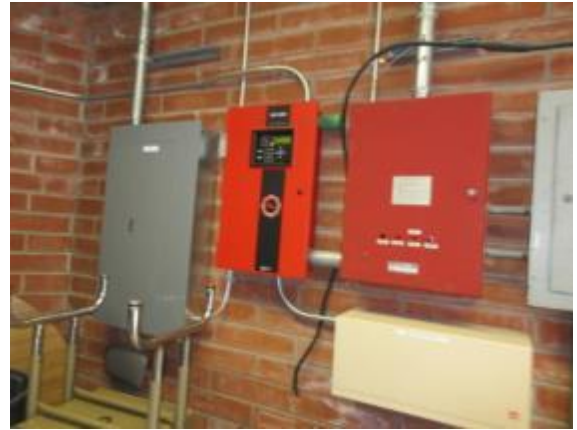
Photo #26: Fire alarm panel
