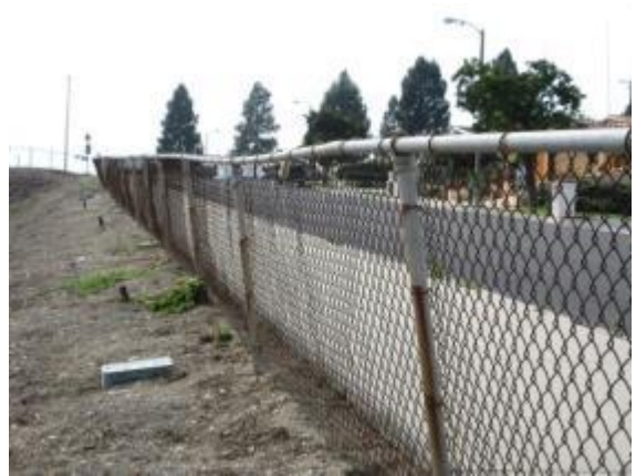
Photo #46: West property fence that is leaning
