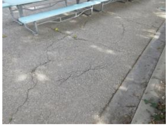
Photo #44: Cracks on asphalt pavement around modular classrooms
