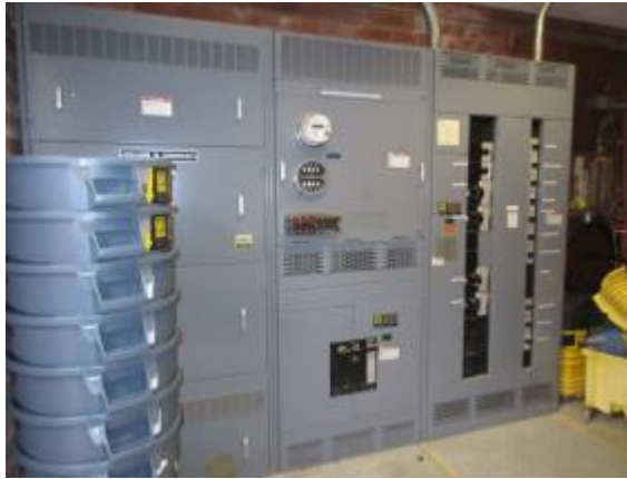
Photo #25: Main electrical switchgear
