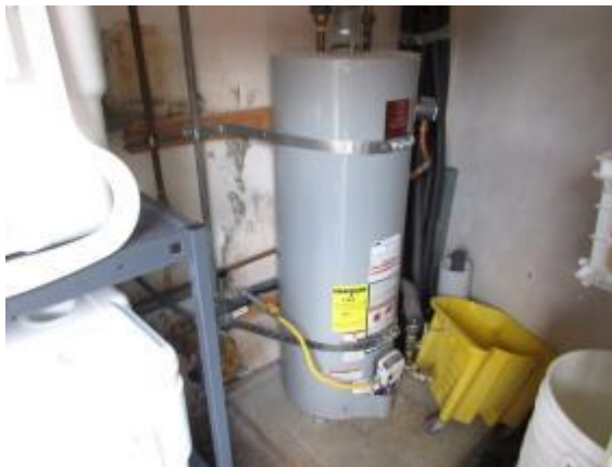
Photo #27: Water heater
