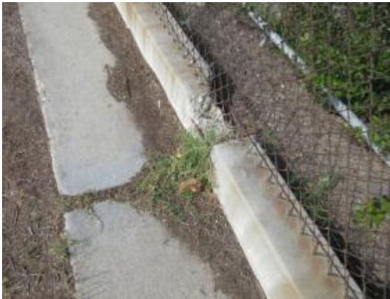
Photo #45: Cracks on curb at east property fence
