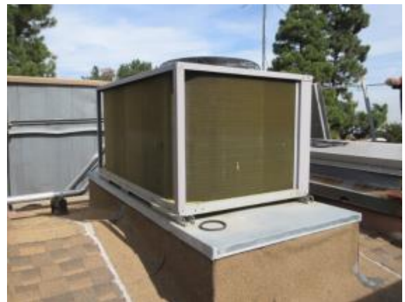
Photo #30: Condensing unit
