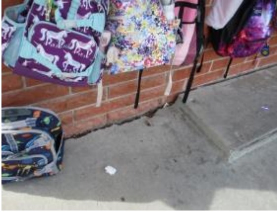
Photo #43: Crack at concrete due to settlement
