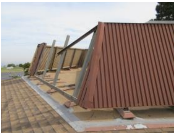
Photo #47: Damaged architectural roof screen
