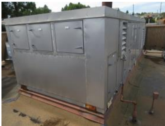
Photo #29: Air handling unit
